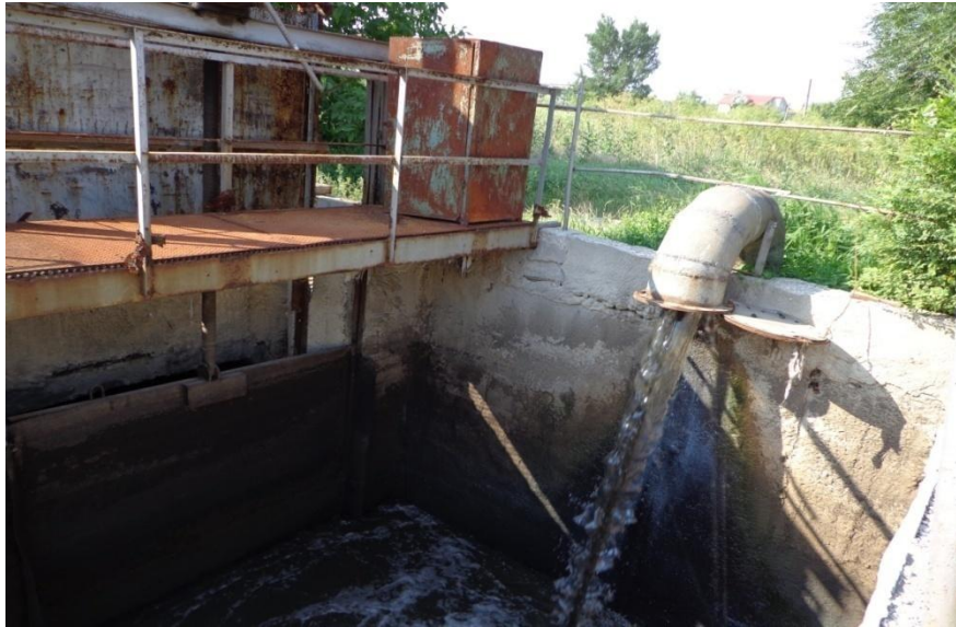
Figure 5. Admission chamber of wastewater at Chişinău Wastewater Treatment Plant
