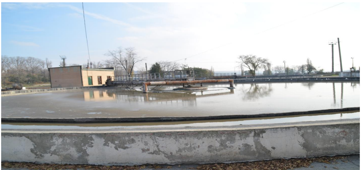
Figure 8. Primary clarifier at Chisinau Wastewater Treatment Plant
