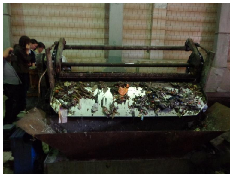
Figure 6. Retentions from screens, Chişinău Wastewater Treatment Plant
