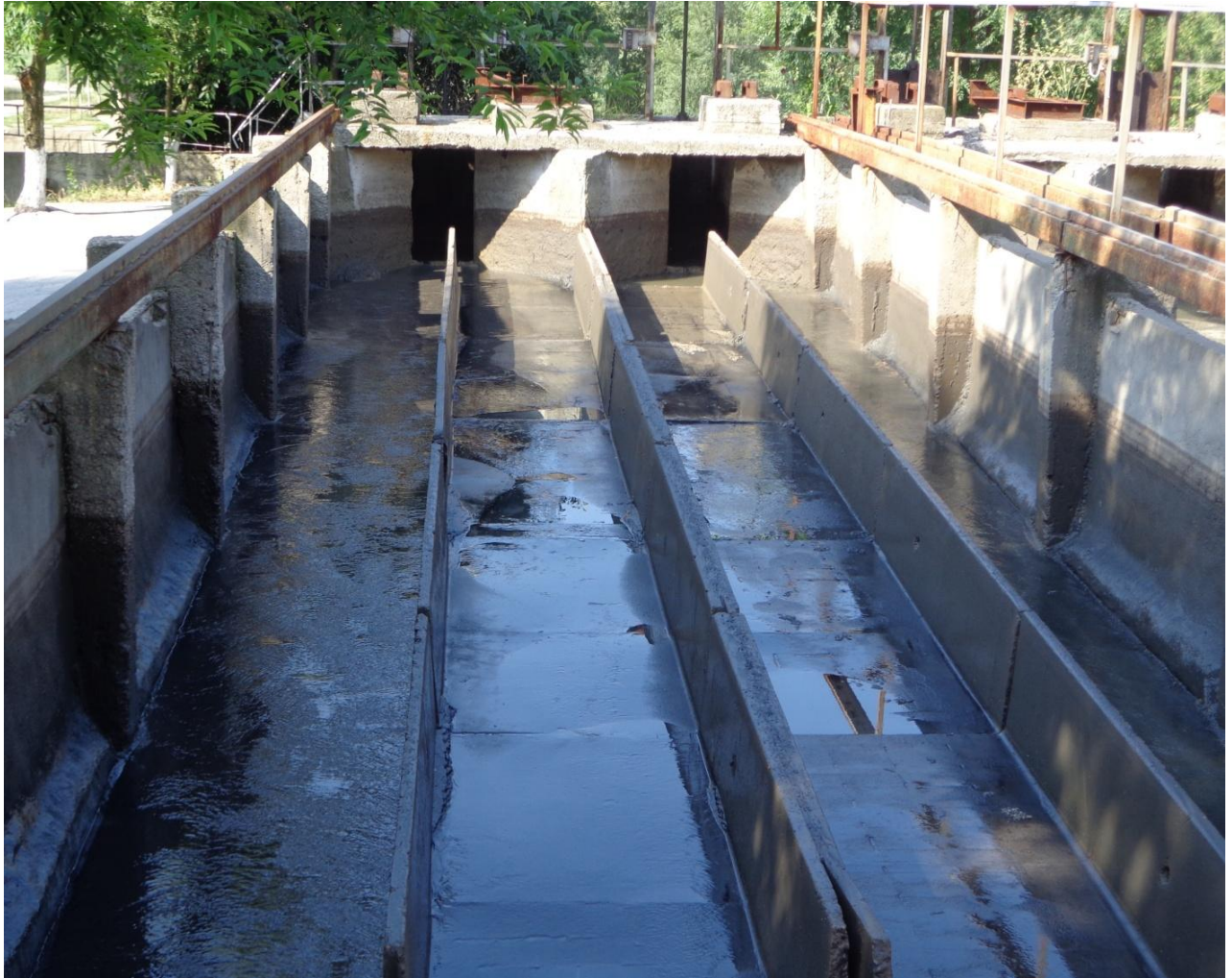
Figure 7. Degritters from Chisinau Wastewater Treatment Plant
